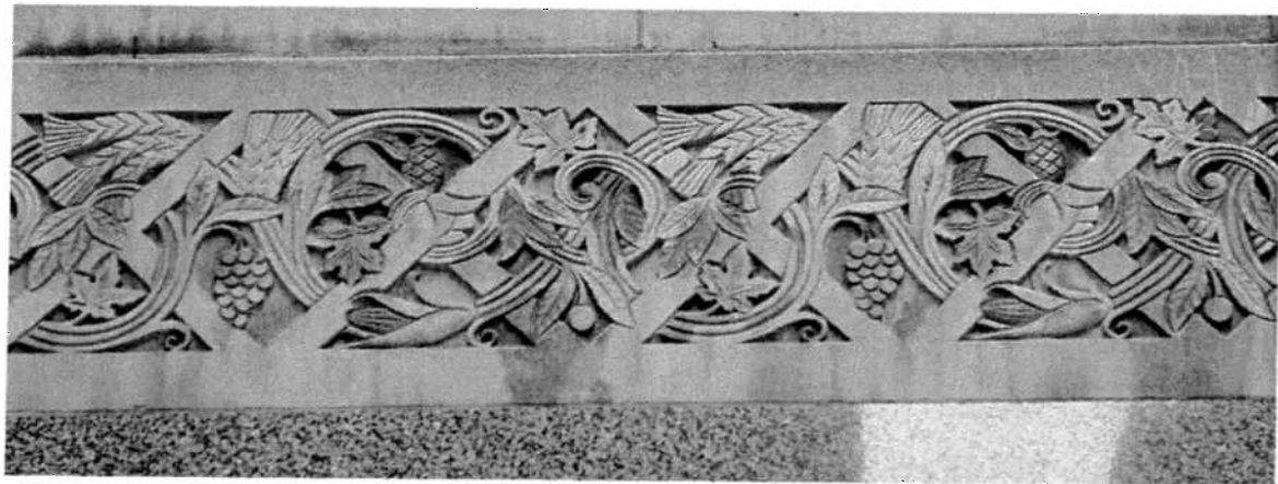
The building is highly decorated with low-relief Art Deco-style ornament executed in both stone and metal. Top: A balconette on the west facade. Middle: A metal spandrel on the east facade. Above: The band of stylized foliate ornament that runs across the top of the building's first floor.
